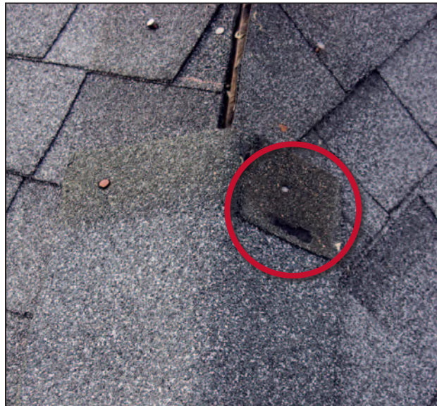
Figure 11-35. Inadequate sealing of the self-sealing adhesive at a hip as a result of the typical hip installation procedure. Estimated wind speed: 105 mph. Hurricane Katrina (Mississippi, 2005)
