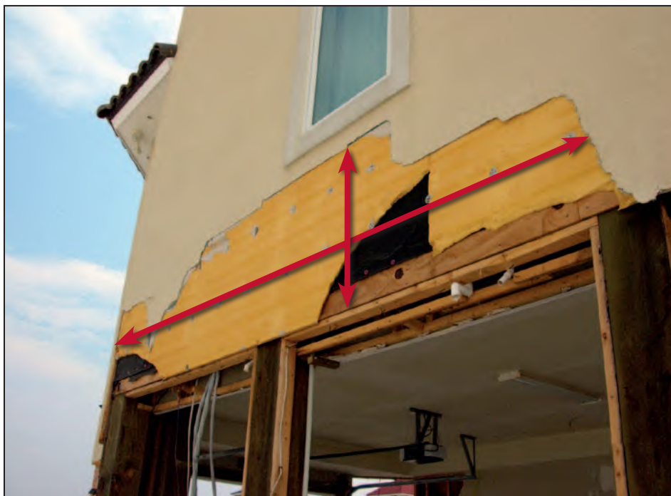
Figure 11-20. Collapse of the breakaway wall, resulting in EIFS peeling. A suitable transition detail at the top of breakaway walls avoids the type of peeling damage shown by the arrows. Estimated wind speed: 105 to 115 mph. Hurricane Ivan (Alabama, 2004)
