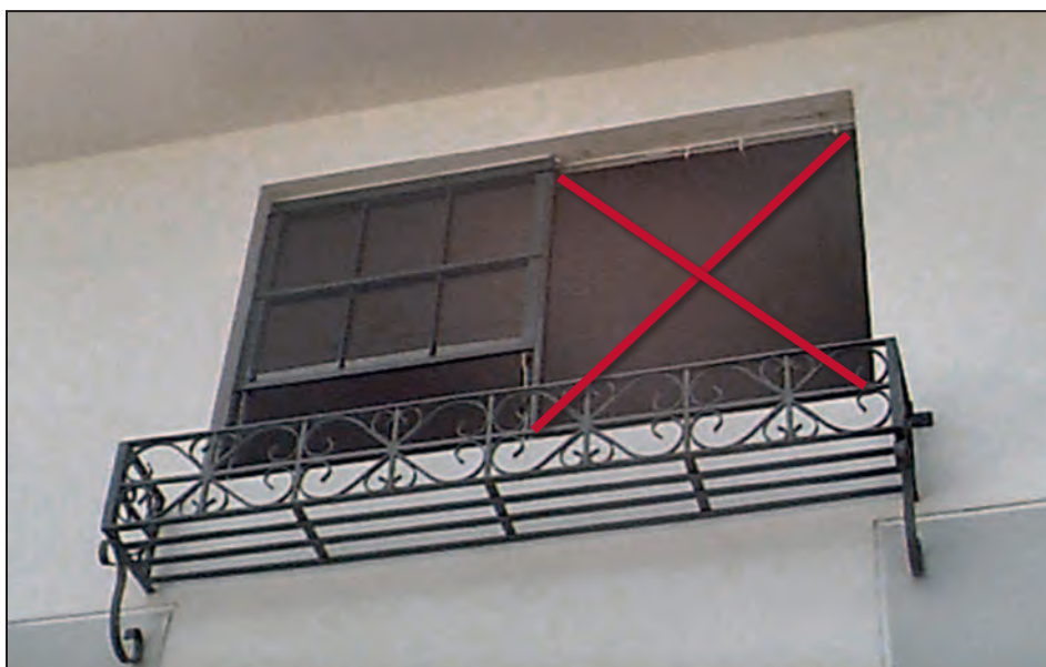
Figure 11-8. Window frame pulled out of the wall because of inadequate window frame attachment. Hurricane Georges (Puerto Rico, 1998)
