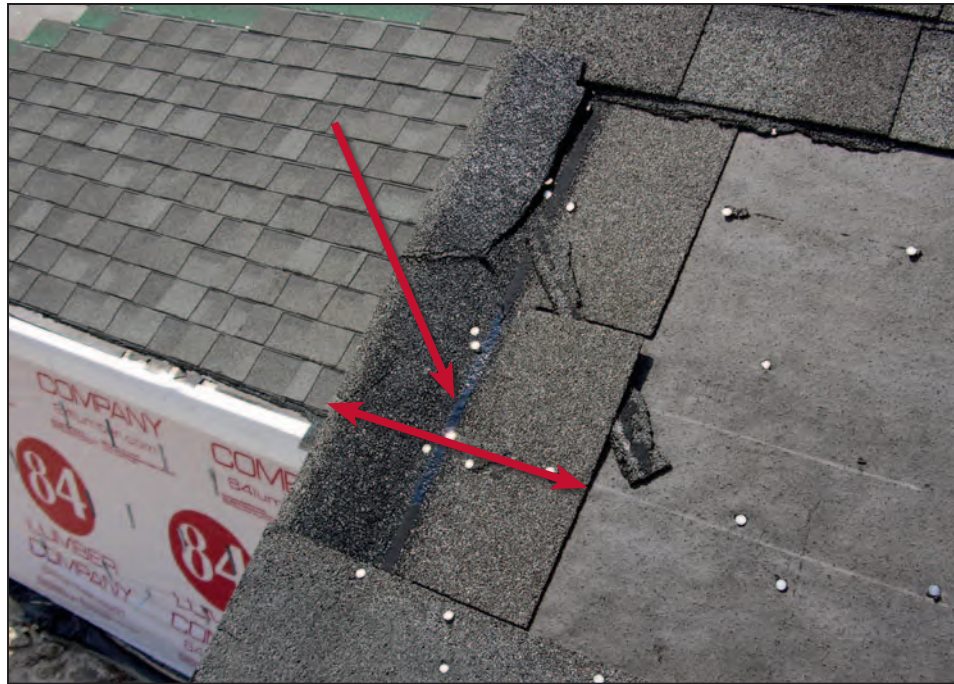
Figure 11-34. A bleeder strip (double-arrow) that was used at a rake blow-off; lack of contact between the tab of the overlying shingle and the bleeder's self-seal adhesive (upper arrow). Estimated wind speed: 125 mph. Hurricane Katrina (Mississippi, 2005)
