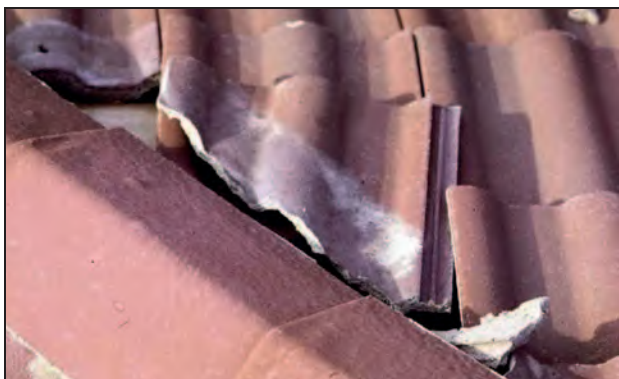
Figure 11-51. Tile that slipped out from under the hip tiles. Northridge Earthquake (California, 1994)
