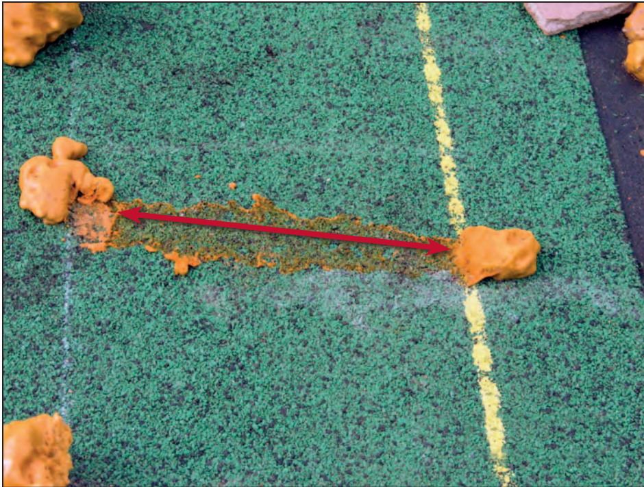
Figure 11-44. Adhesive that debonded from the cap sheet
