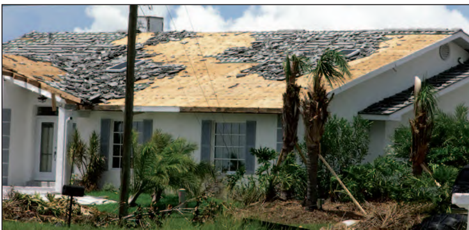
Figure 11-40. Large area of blown-off underlayment on a mortar-set tile roof. The atypical loss of waterproofing tile underlayment resulted in substantial water leakage into the house. Estimated wind speed: 140 to 160 mph. Hurricane Charley (Florida, 2004)
