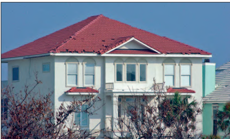
Figure 11-39. Blow-off of eave and hip tiles and some broken tiles in the field of the roof. Hurricane Ivan (Alabama, 2004)
