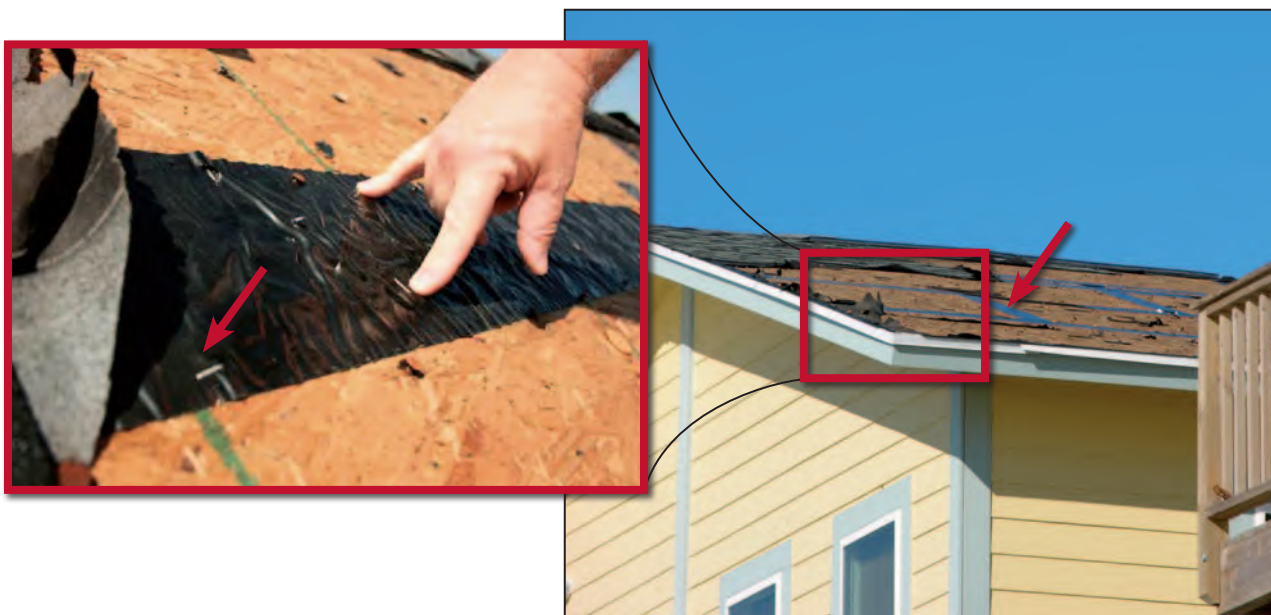
Figure 11-28. House that used enhanced underlayment Option 3 with taped sheathing joints (arrow). The self-adhering modified bitumen tape (inset) was stapled because of bonding problems. Estimated wind speed: 110 mph. Hurricane Ike (Texas, 2008)
