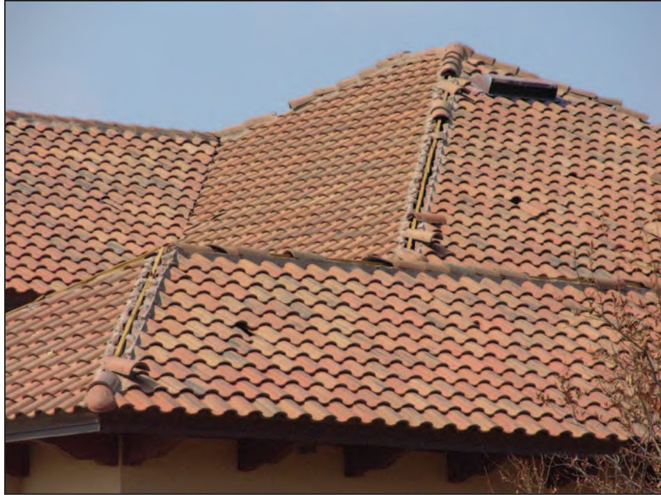
Figure 11-46. Blow-off of hip tiles that were nailed to a ridge board and set in mortar. Hurricane Ivan (Florida, 2004)
