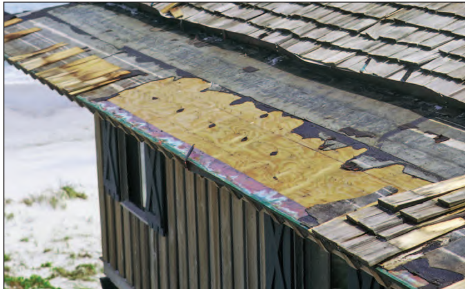
Figure 11-54. Loss of wood shingles due to fastener corrosion. Hurricane Bertha (North Carolina, 1996)
