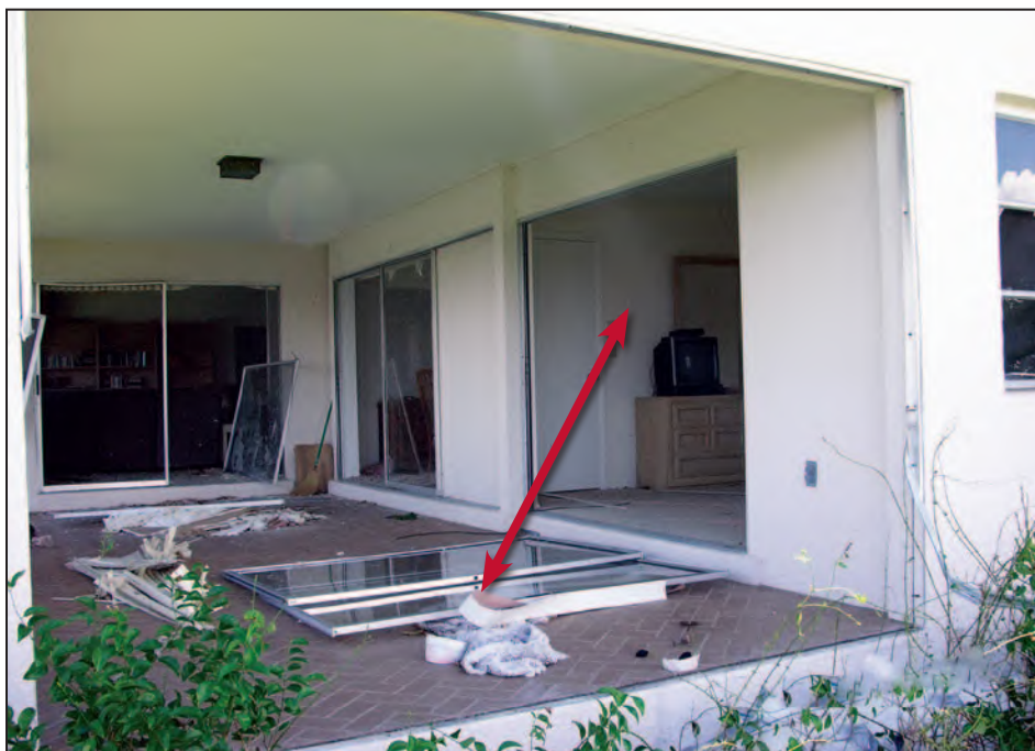
Figure 11-5. Sliding glass doors pulled out of their tracks by wind suction. Estimated wind speed: 140 to 160 mph. Hurricane Charley (Florida, 2004)
