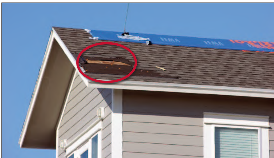
Figure 11-31. Loss of shingles and underlayment along the rake. Estimated wind speed: 110 mph. Hurricane Ike (Texas, 2008)
