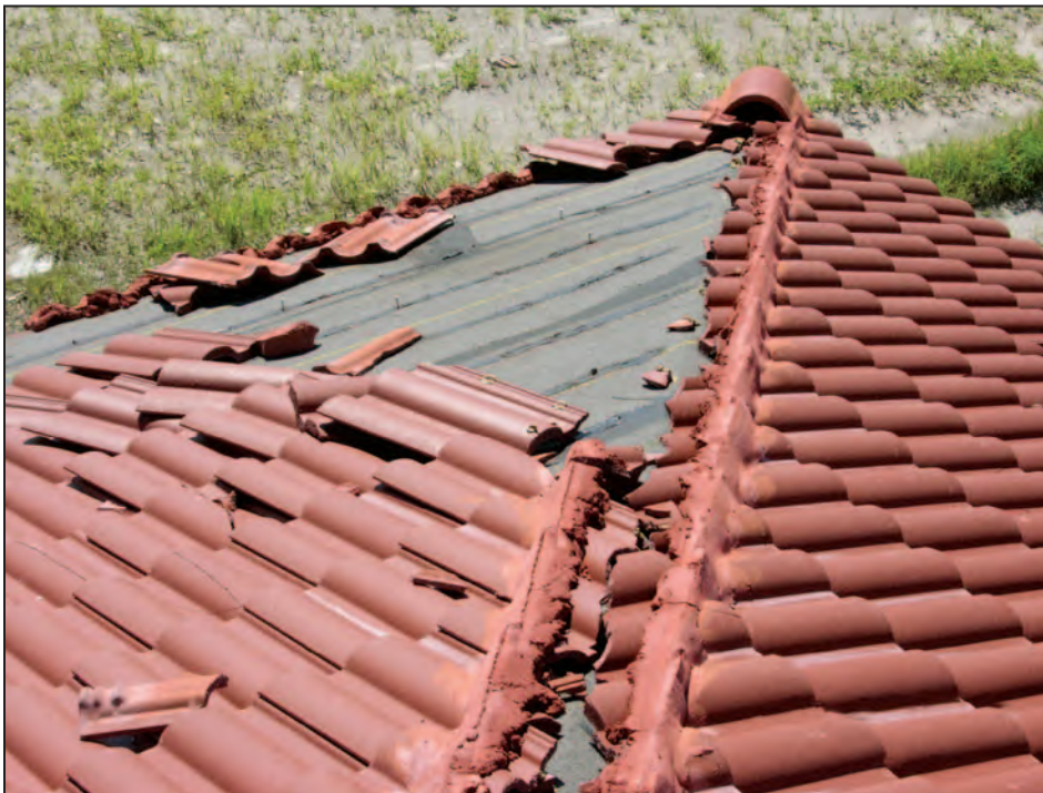
Figure 11-45. Blow-off of mechanically attached tiles. Estimated wind speed: 140 to 160 mph. Hurricane Charley (Florida, 2004)
