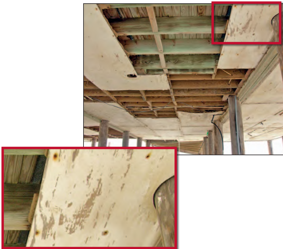
Figure 11-4. Plywood panels on the underside of a house that blew away because of excessive nail spacing. Note the corroded nails (inset). Estimated wind speed: 105 to 115 mph. Hurricane Ivan (Alabama, 2004)
